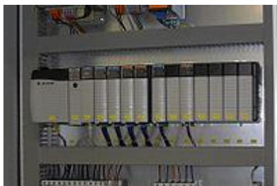
Allen-Bradley PLC installed in a control panel
